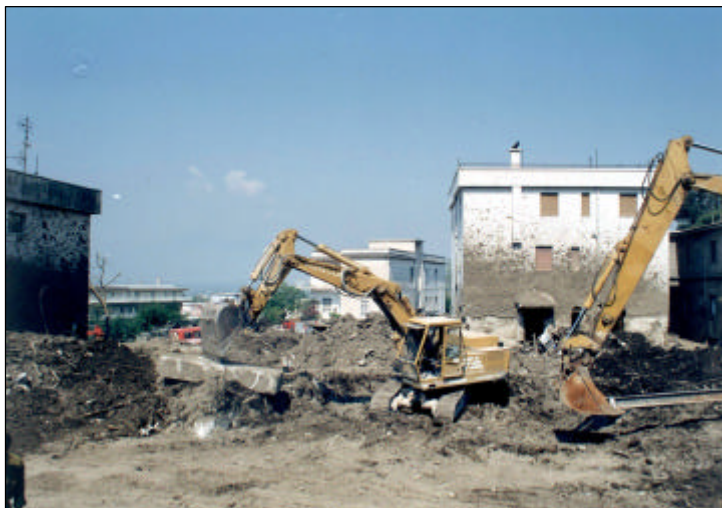
Figure 2.4 Excavators in action during the response phase in Sarno. In the lower picture, the grey bend on the white building, which marks the maximum level reached by the mudflow can be observed (Centro Documentazione, VV.F. Napoli).
