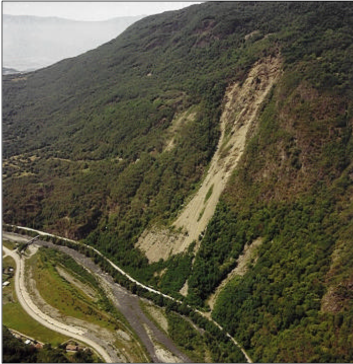
Figure 8.2 View of the central and lower part of the unstable slope at Les Ruines de Séchilienne. The lighter area corresponds to shallow movements (topples and rockfalls). The Romanche River and the diverted road are apparent at the bottom
