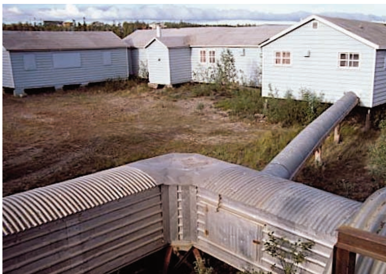
Inuvik can expect foundation damage from thawing permafrost in up to 75% of its existing buildings. Supporting infrastructure such as the “utilidors” (foreground) will also be impacted. (Jerry Peek)
