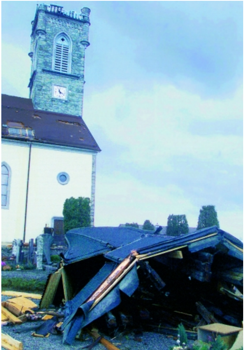
The parish church at Attalans (Switzerland) shows the whole spectrum of storm losses, from the small losses characteristic of windstorm (such as tiles) to the more unusual large losses (church spire).
