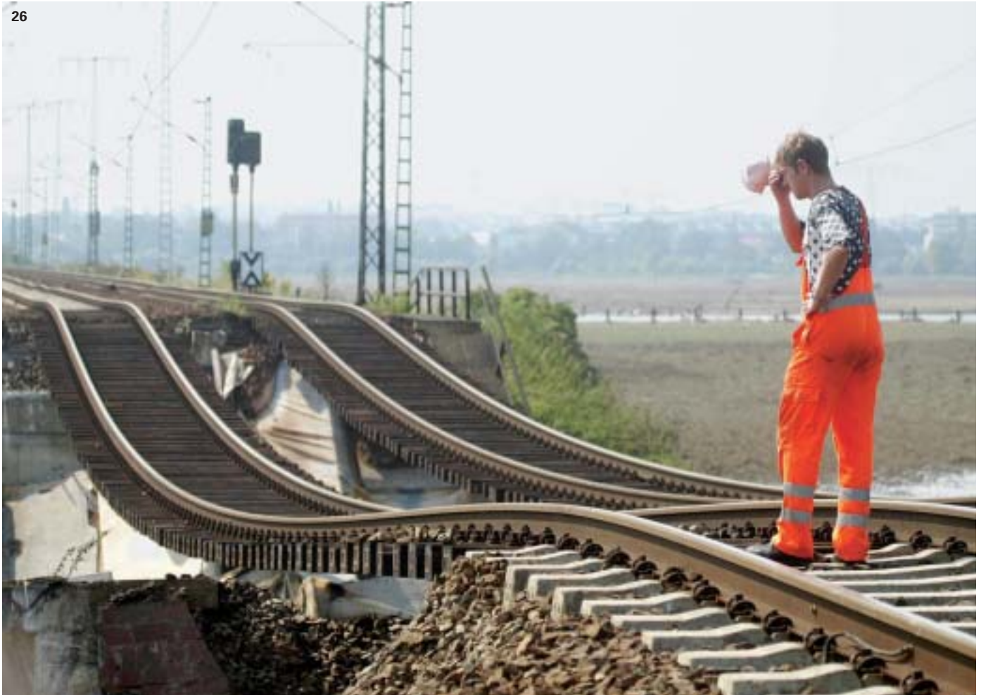
26 State buildings and infrastructure are often not insured. In principle cover is available for railway tracks (CECR: civil engineering completed risks), but many countries do not take advantage of it. In the great summer floods many railway lines in the Czech Republic, Austria, and Germany were badly damaged.
