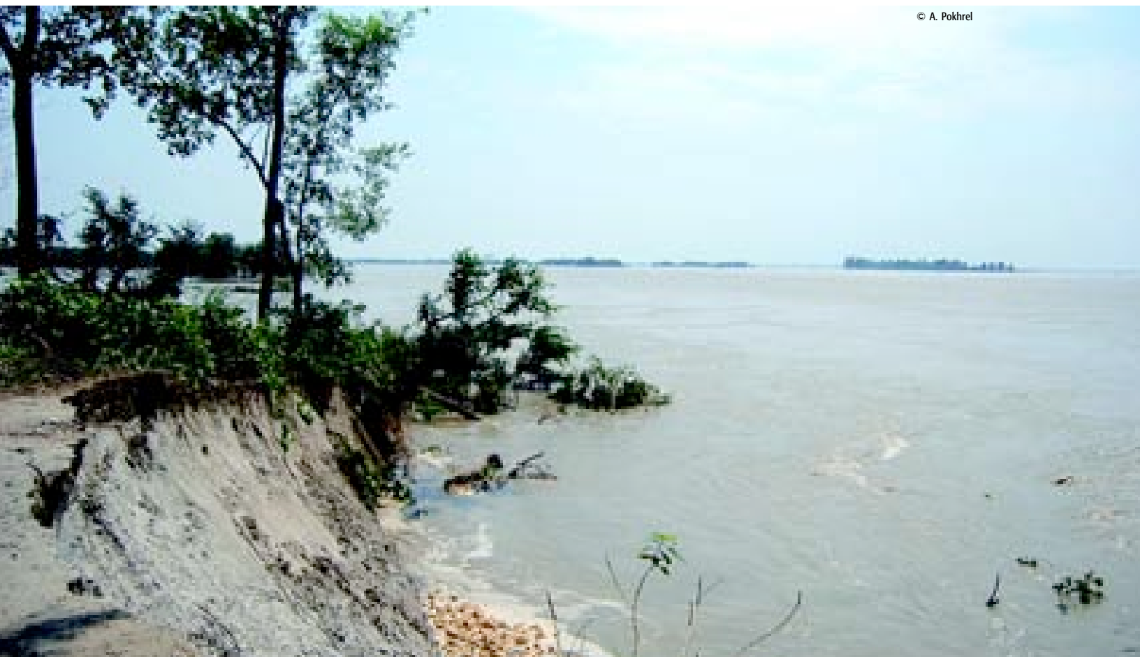
FIGURE 5 | August 18, 2008 Kosi embankment breach site at Paschim Kusaha, Nepal
