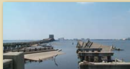
Hurricane Katrina damage to bridge
