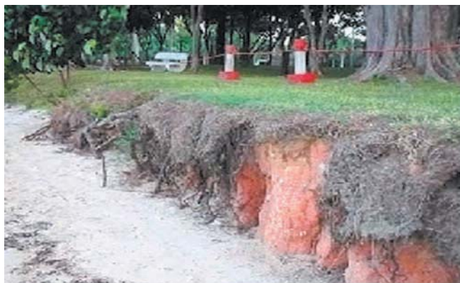
Figure 3.10. Coastal Erosion at East Coast Park, Singapore
