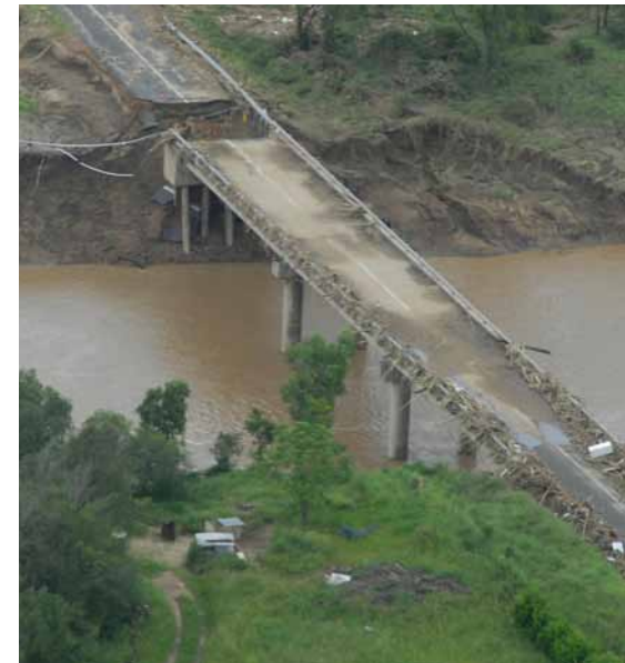
Photo: Flood damage after the Toowoomba flood disaster, January 2011. © APN Regional Media
