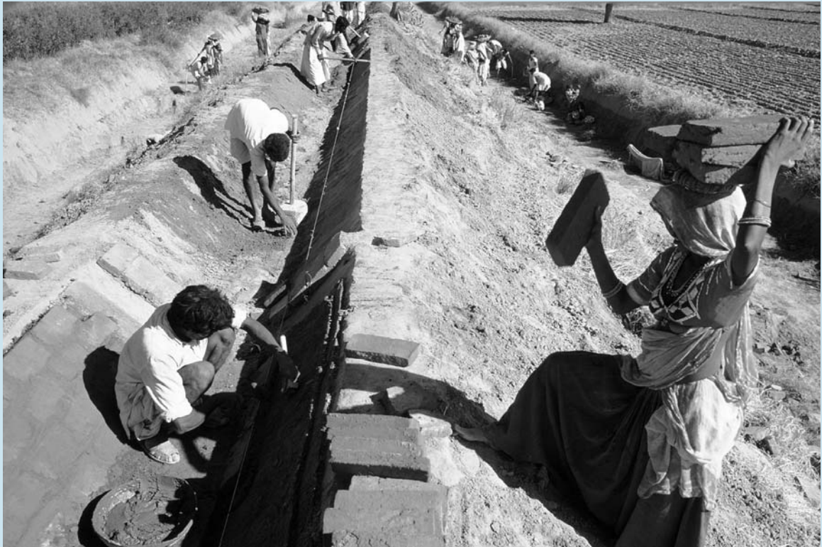
Building a canal for irrigation in India. Photo by Ray Witlin, courtesy of World Bank Photo Library.
