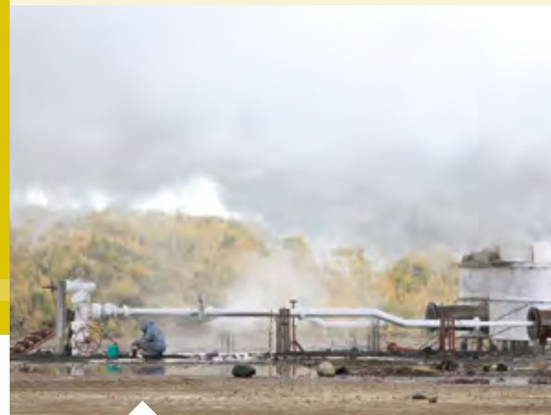
$25 million from the SREP managed by the AfDB is helping to finance Kenya's Menengai geothermal power project, which is structured as a PPP and aims to produce electricity for 500,000 households and displace 2 million tons of CO 2 emissions annually. Photo: Africa Express
